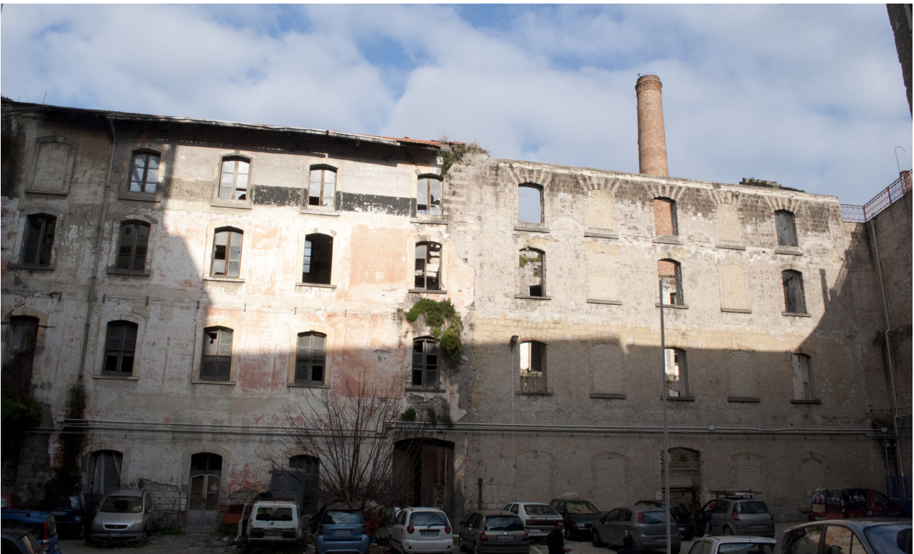
Figure 9. The Garofalo pasta factory at present with the interior floors collapsed, by courtesy of Francesco Paolo Longobardi.
