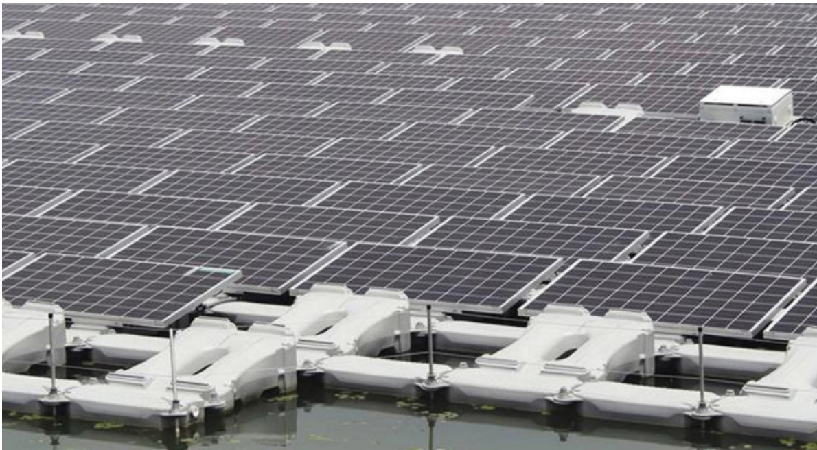
Figure 4. Panels at the Bordentown Avenue Water Treatment Facility. Source: www.wateronline.com .
