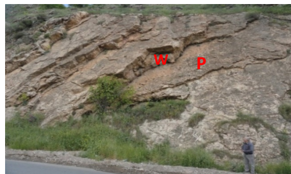
Figure 5. Showing the plane sliding (P), and the wedge sliding (W) at station 1.
