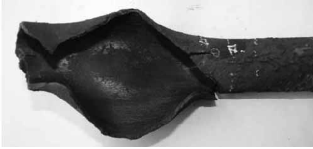
Fig. 6. Failure of the tube Rys. 6. Awaria rurociągu
