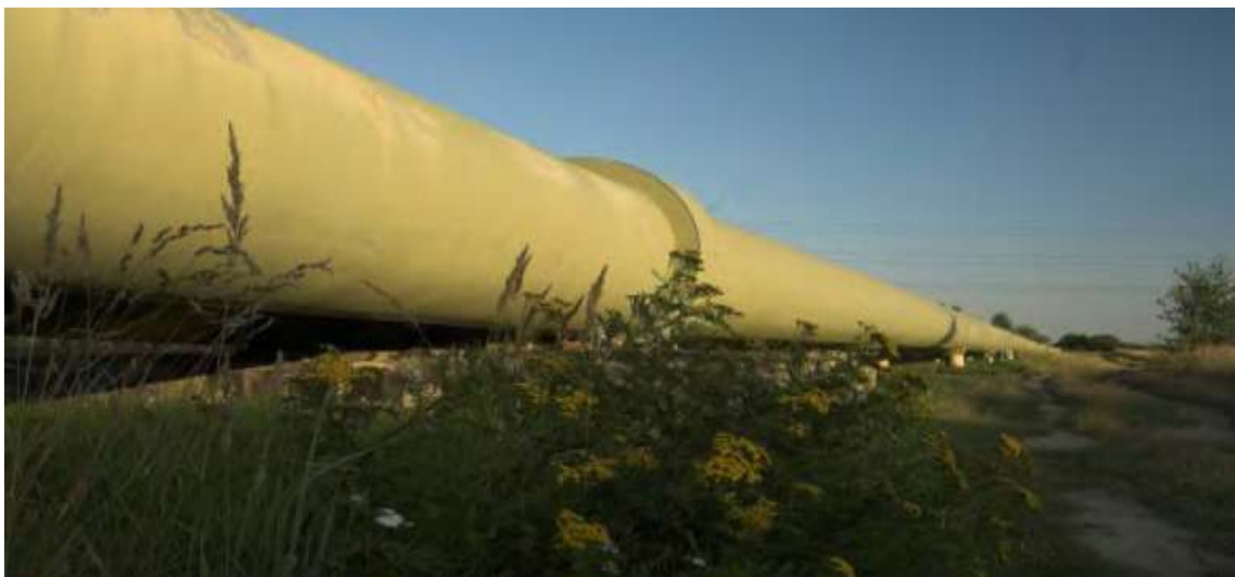
Figure 11. Pipes for transporting large-scale heat (2xDN 1200) between Melnik and Prague [30]
