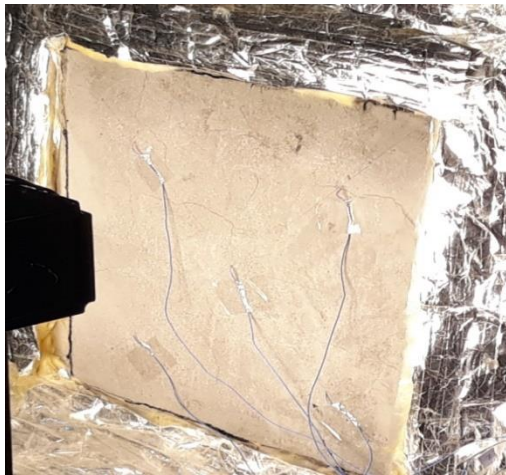
Figure 6. Install sensors on both sides of the wall and in the middle of the room
