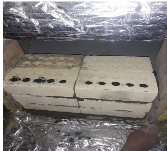
Figure 9. Put the tire scrap power in the line of the outer holes during construction
