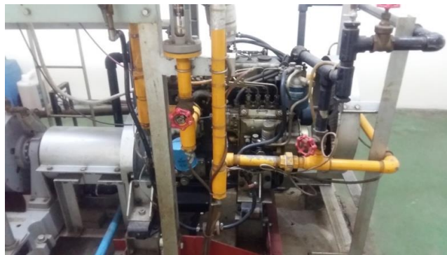
Fig. 2. The condition of the diesel engine observed
