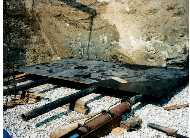
Fig. 4. Installation of the steel plate forming the base of the large-scale lysimeter. The steel plate was inserted by four hydraulic piston rods into the wall of the excavation at 3.3 m depth.
