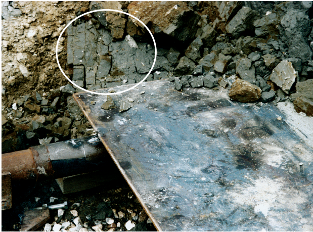
Fig. 2. Clayey till as seen at 3.3 m depth at the Avedøre field site. Two vertical and one horizontal fracture systems give the till a brick-like appearance. The steel plate forms the bottom of the lysimeter.
