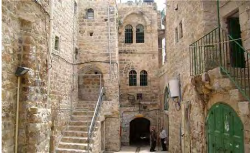
Figure 4. The bad situation of some houses in the old town of Jerusalem.
