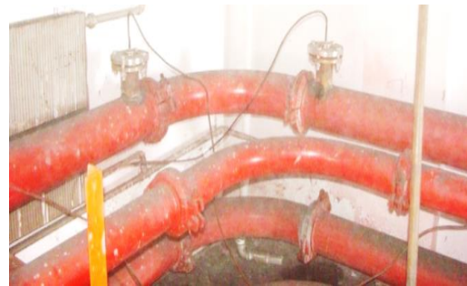
Figure 2: Two sensors collecting local resistance loss data in bent pipe
