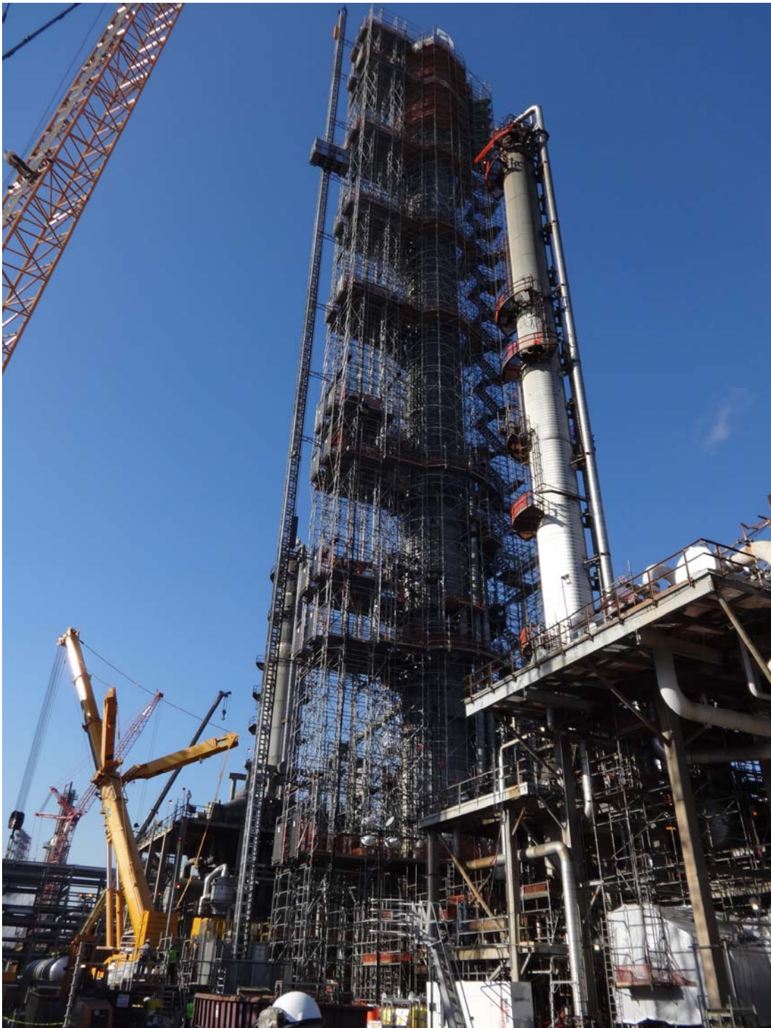
Figure 3: C 2 Splitter being Revamped – Note the construction Elevator attached to the Vessel
