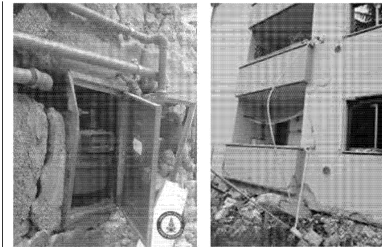
Figure 4 Damage on gas pipelines caused by heavy damage to stone walls (at left) and of RC (at right) residential buildings
