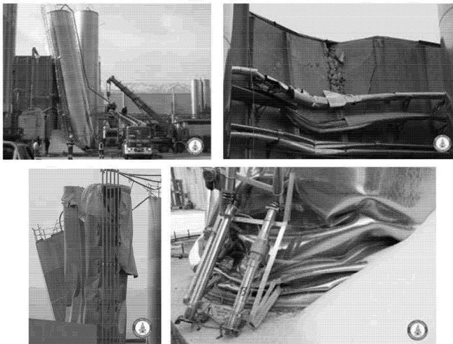
Figure 2. Damages to, and caused by, silos at VIBAC facility in the Bazzano industrial area, 7 km South of L'Aquila town.
