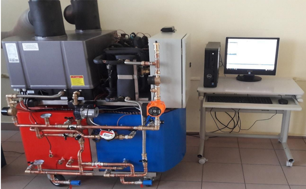
Figure 1: Installation of a DHW heat pump in a test stand
