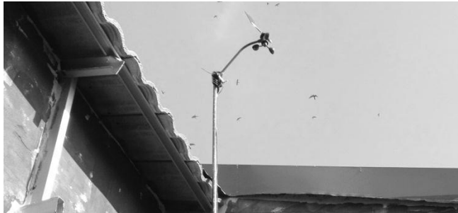
Figure 3: Anemometer (as part of Weather station) is placed on the roof top
