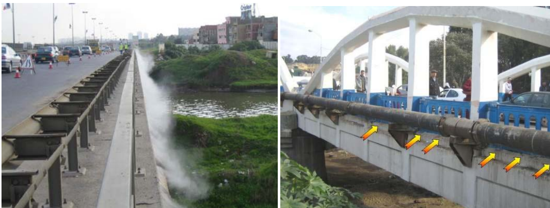
Figure 1: Views of the main areas of application of masking agents on the highway bridge and on the main pedestrian bridge
