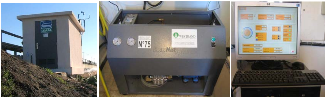
Figure 3: Views of the technical booth with the high pressure spraying station and PLC control
