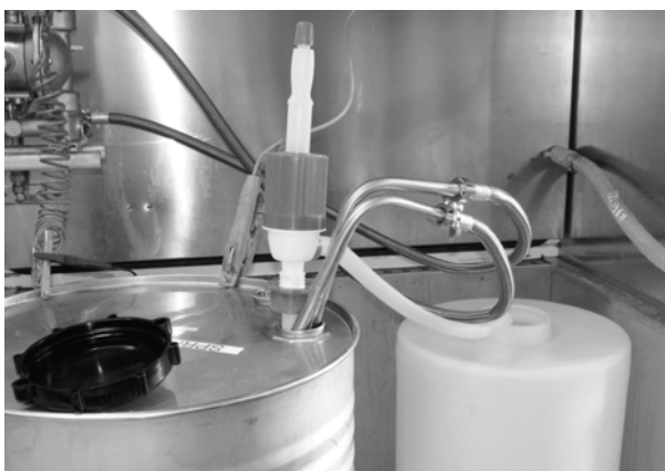
Figure 1, Filling with manual plastic pump from 200 l metal drum to 120 l plastic container
