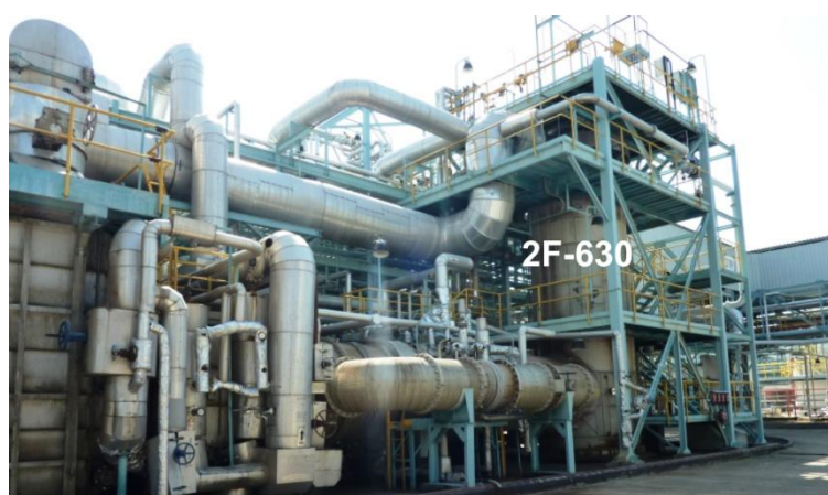
Figure 1: Incineration unit 2F-630 at Momentive Specialty Chemicals, Inc. in Sokolov
