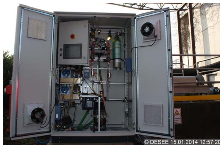
Figure 3: SOU installed in Hannover
