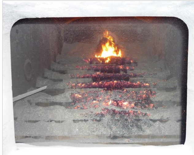
Figure 3: Fuel and ashes layer in 2.5 MW boiler operated at ca. 0.2 MW
