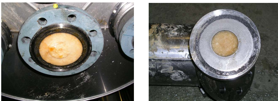
Figure 4: Plugged Reactor Inlet C 400 (left) and Plugged Reactor Feed Line (right)
