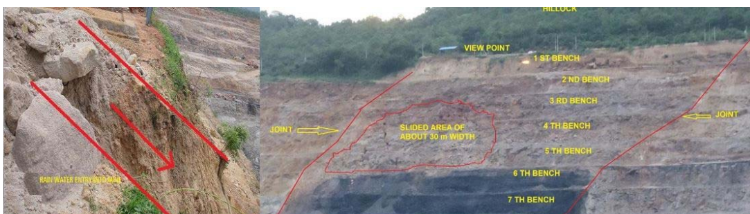
Figure 9: Photograph depicting failure and displacement in Goutham Khani Opencast Project
