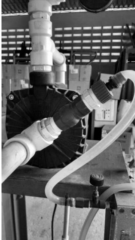
Figure 4: Adapter installed at the inlet of the centrifugal pump.
