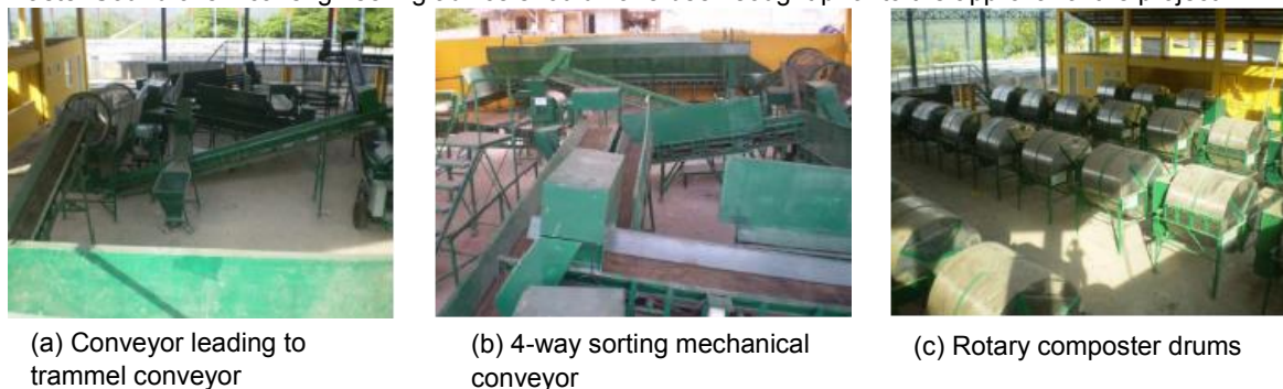
Figure 1: Sets of solid waste sorting equipment and rotary bioreactors at the CMRCF
