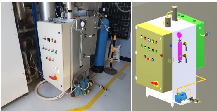
Figure 2: The real steam boiler (<10bar) and the virtual twin exploited in the training system
