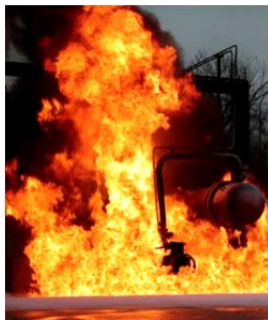
Figure 7: Petrol leak fire
