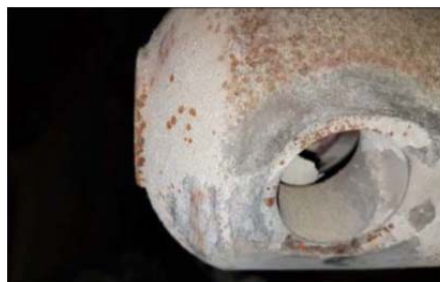
Figure 8: lance head of soot blower shows signs of wear.
