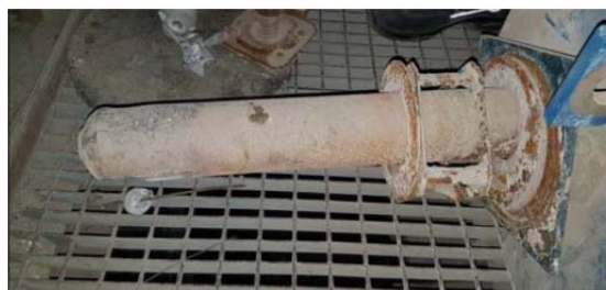
Figure 7: soot blower after removal from the furnace.
