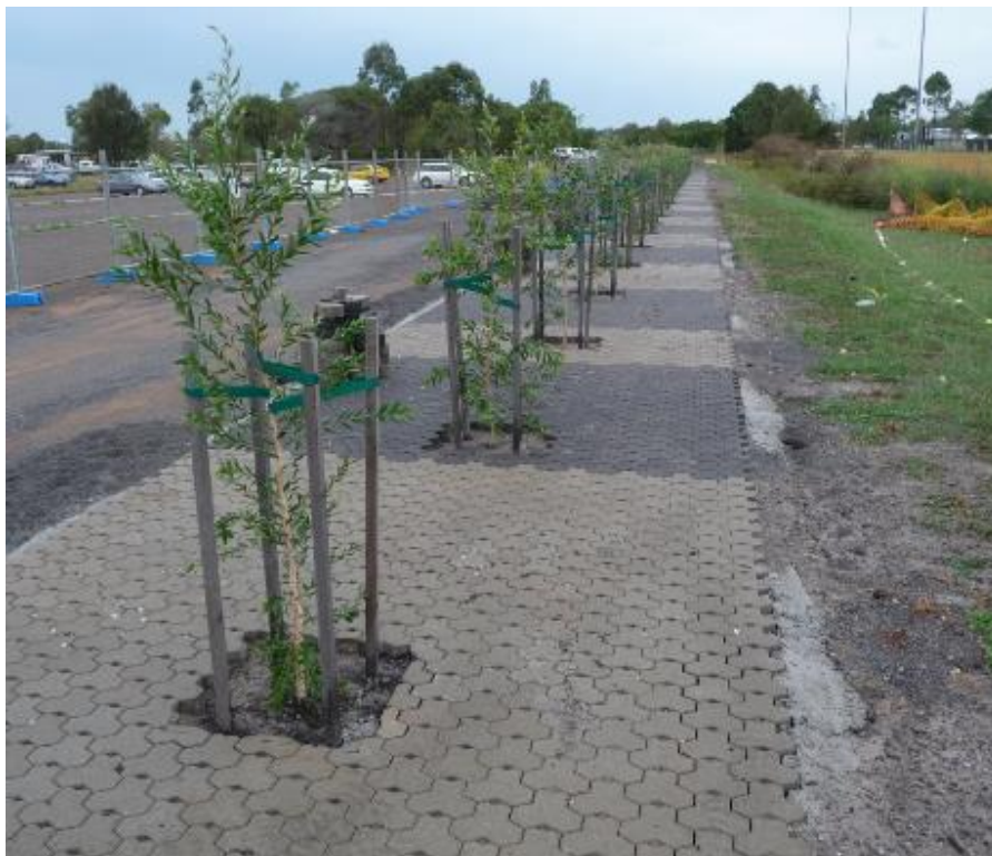
Figure 2: Juvenile street trees soon after planting in a permeable pavement system in Australia
