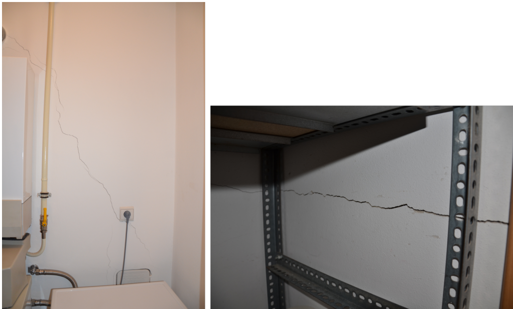
FIGURE 1. Cracks in partition walls.
