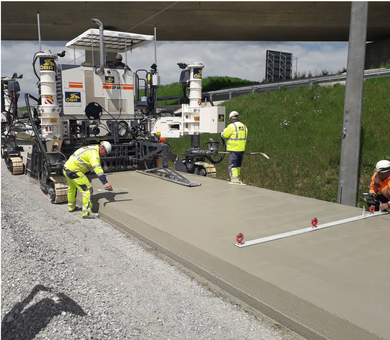
FIGURE 2. Machine laying by finisher of the hydraulically bound layer under the top concrete slab (HGT), Photography author: DB Projekt Stuttgart-Ulm GmbH/Ondřej Tomaschko
