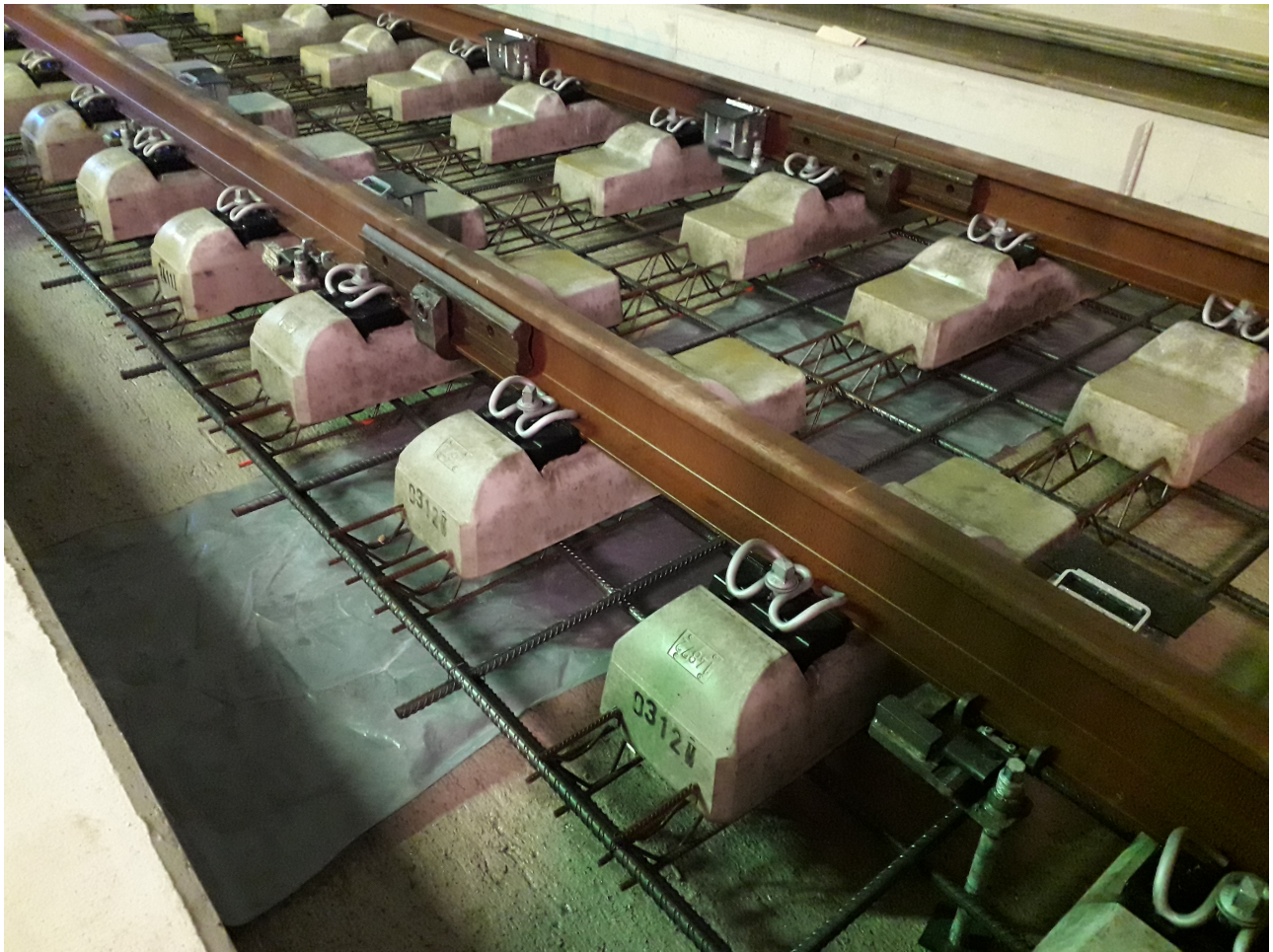
FIGURE 1. Ballastless track type RHEDA 2000 before casting (by concrete), photography author: DB Projekt Stuttgart-Ulm GmbH/Ondřej Tomaschko
