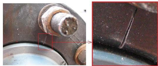
FIGURE 2. Crack and crack detail.
