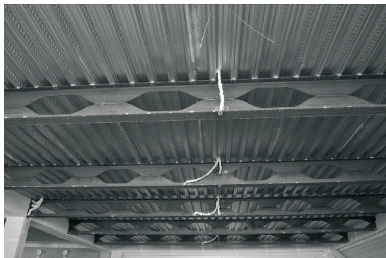
Fig. 5: Thermocouples for gas and steel temperatures
