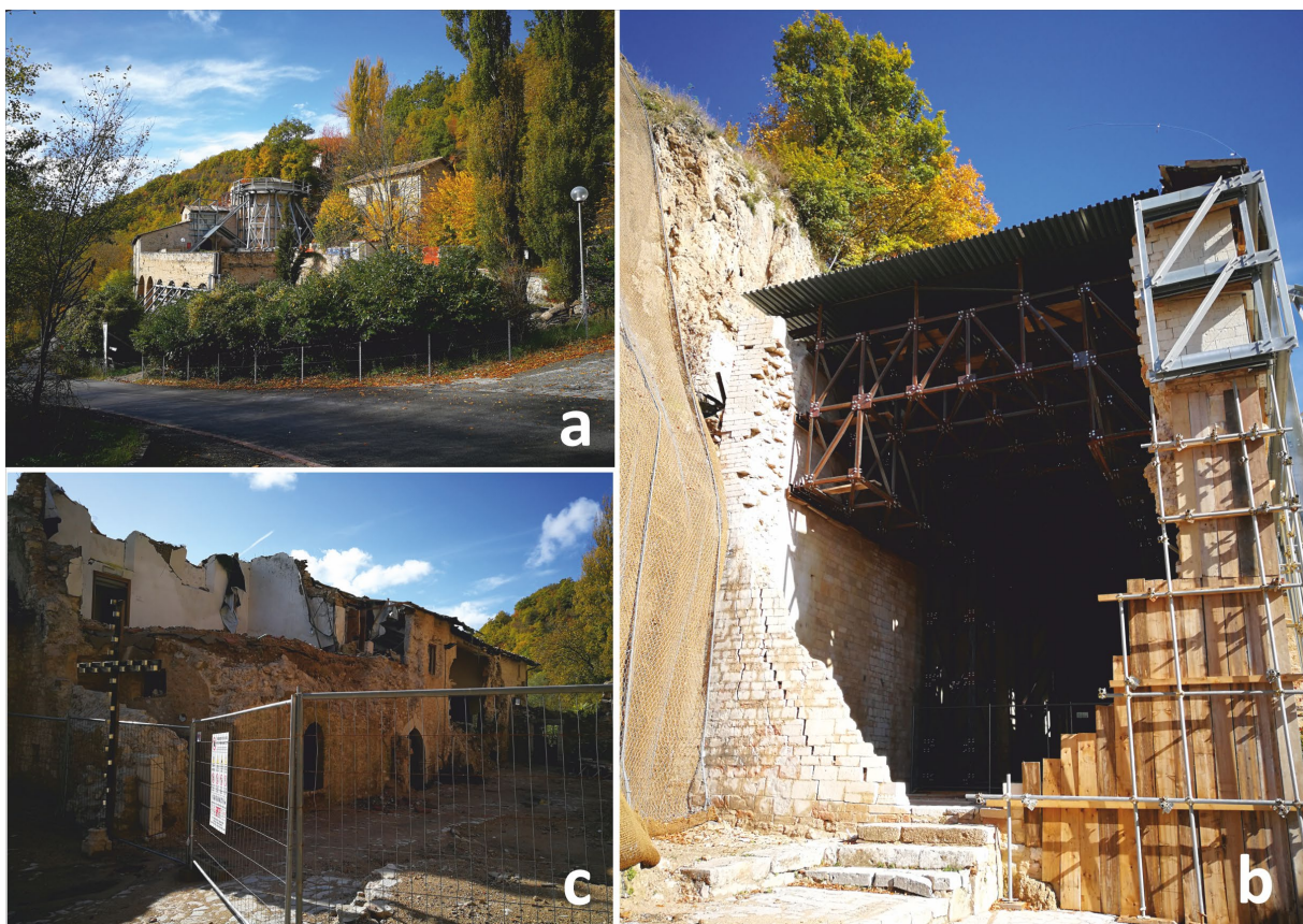
Figure 1. (a) View of the Sant'Eutizio Abbey partially collapsed owing to shaking and seismically triggered landfall; The figures (b) and (c) show the church and building severely damaged, respectively.
