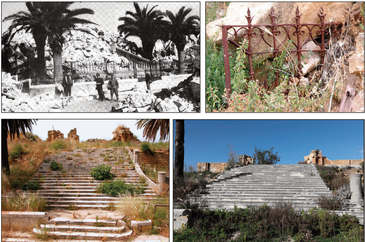
Figure 8. Salaparuta, degradation process of the Holy Mother church. Some architectonic details, such as the railings, balustrade and entrance steps are now definitively lost.
