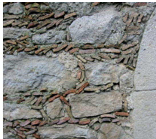
FIGURE 13. Naso (Me), masonry palimpsest with earthenware used to fill lesions
