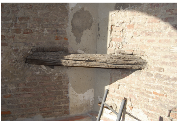
FIGURE 20. Wooden chain inserted in an internal corner of the belfry of the Church of San Lorenzo in Borgo San Lorenzo (FI).
