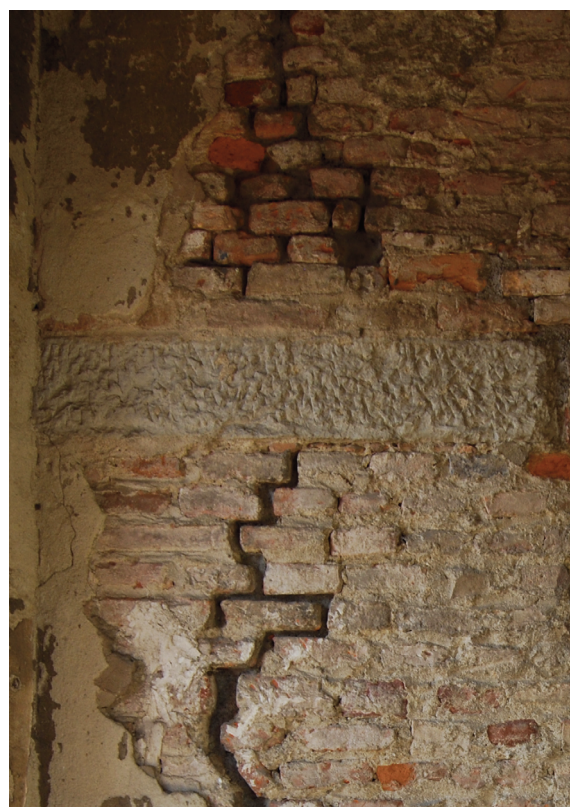
FIGURE 21. Limestone chains inserted in some internal stonework of the belfry of the Church of San Lorenzo in Borgo San Lorenzo (FI).
