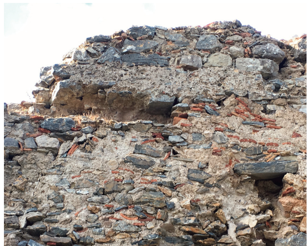
FIGURE 12. Gioiosa Guardia (Me), wooden beam drowned in the masonry.
