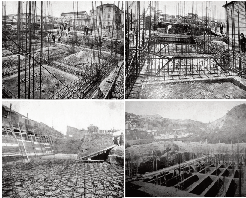
FIGURE 6. The types of structures for “anti-seismic” foundations realized for the economic houses program managed by the UEM in the first years of the reconstruction: basic rigid frame; detail of the concrete steel foundations; reinforced concrete bed; slabs of hollow foundations. [Unione Edilizia Messinese, 1917]
