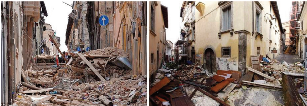
FIGURE 5. Interruption of road sections due to the seismic vulnerability of the buildings facing the street (L'Aquila, 2009).
