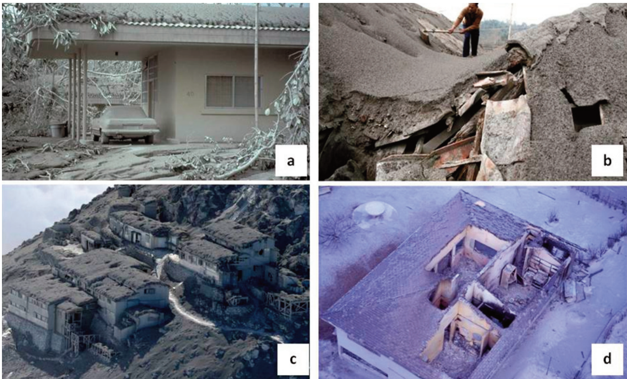
FIGURE 4. Roof vulnerability to ash fall: a) 1991 eruption of Mount Pinatubo, Philippines ( www.volcanoes.usgs.gov ); b) 2014 eruption of Mount Kelud, Indonesia (AFP photo); c) 2014 Mount Ontake eruption, Japan (Photo / Kyodo News); d) 1997 eruption of the Soufriere Hills, Montserrat, UK.
