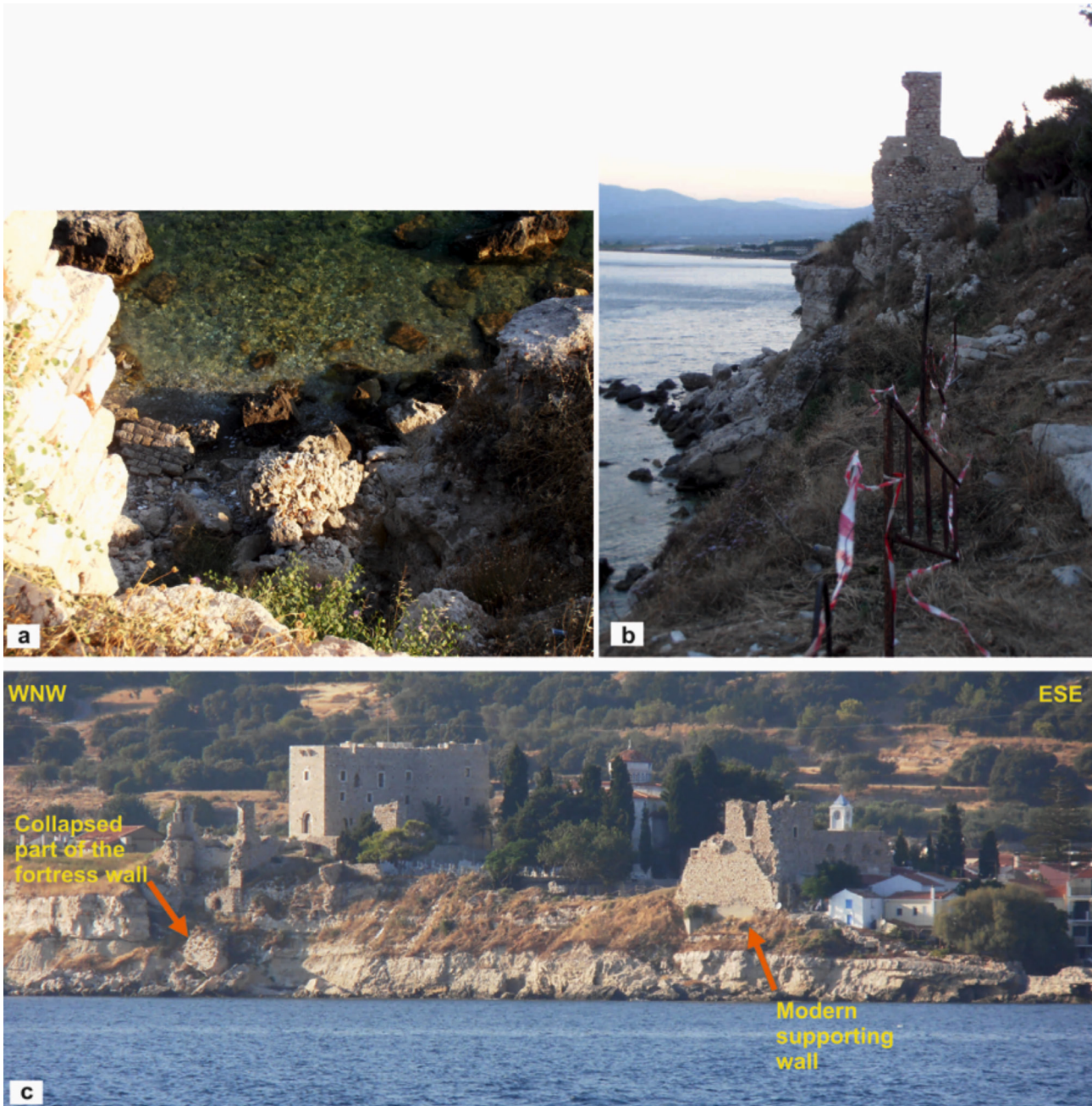
Figure 5. Slope instabilities as recorded on the southern escarpment at Logothetis Castle site (a) collapsed part of the fortress wall along with rock fall debris deposits (b) the active escarpment and the WNW fortress tower with debris deposits, (c) the preserved remains of the WNW and ESE towers of the fortification wall.
