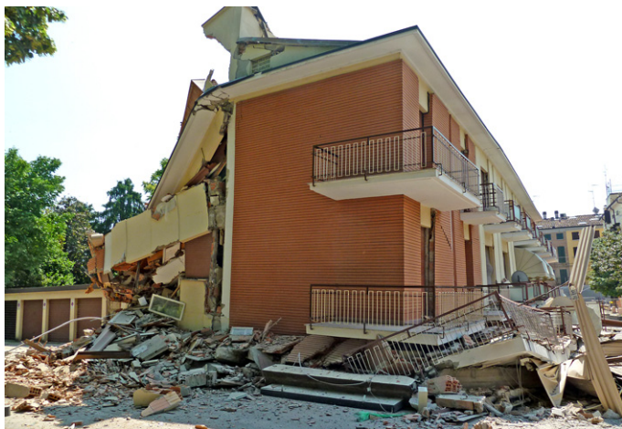
Figure 6. Cavezzo ( I_s 7 MCS). Total collapse of the pilotis of a reinforced-concrete building in the old center (photo taken on the morning of May 29, 2012). This building experienced level 2 damage because of the May 20 mainshock, and was not inhabited when it collapsed on May 29.
