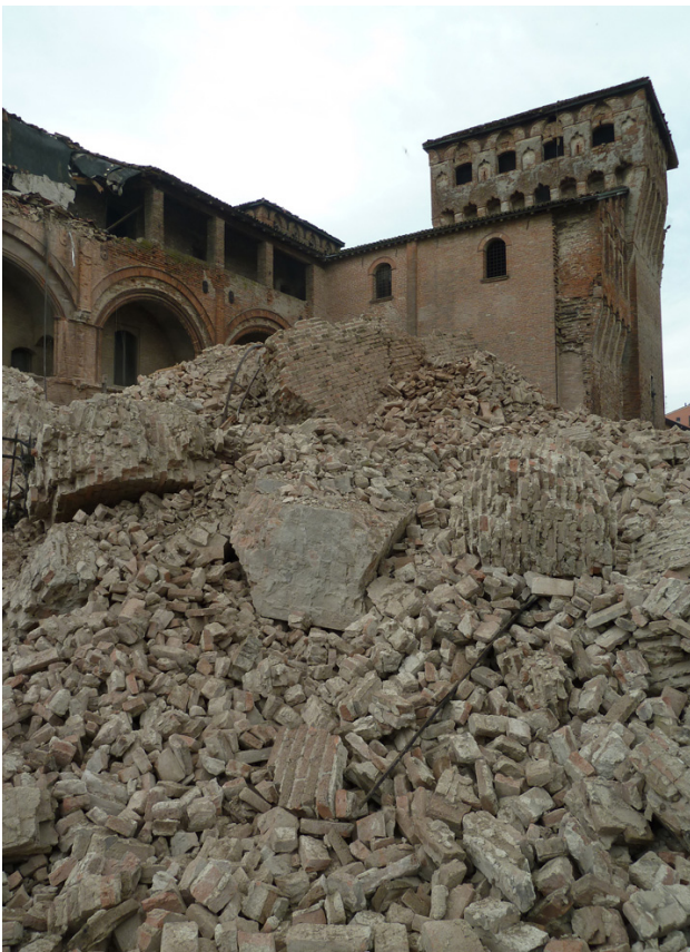
Figure 3. The morning of May 20, 2012. Top: View of the Mirandola Cathedral (15th century). At that time, only a few architectural elements at the top of the façade had fallen down, besides the incipient façade detachment. The church was damaged again, and more seriously, by the May 29, 2012, mainshock. Bottom: Partial collapse of the Estense Castle (15th century) in Finale Emilia.
