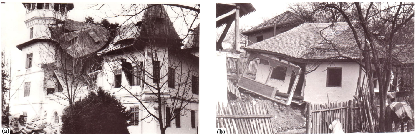
Figure 5. Partial collapse of a masonry building at Drajna (a) and heavy damage to a wooden house at Slon (b), in Prahova county (photos by Pantea [1979]).
