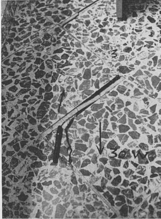
Fig. 5 - A fracture inside a house in Tremestieri (Mt. Etna) along the same alignment as that of Fig. 4 (NNW-SSE) with the displacement prevalently horizontal and clockwise. The cement joint in the floor tiles was made after a previous fracture (about 20 years ago) occurring with the same amount of displacement and analogous phenomenology.
