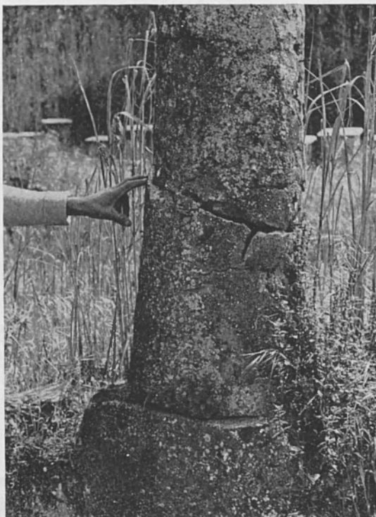
Fig. 2 - A patio column broken and twisted in an anticlockwise direction at Vulcano Piano (the island of Vulcano, Aeolian Islands; earthquake of 15th April 1978).
