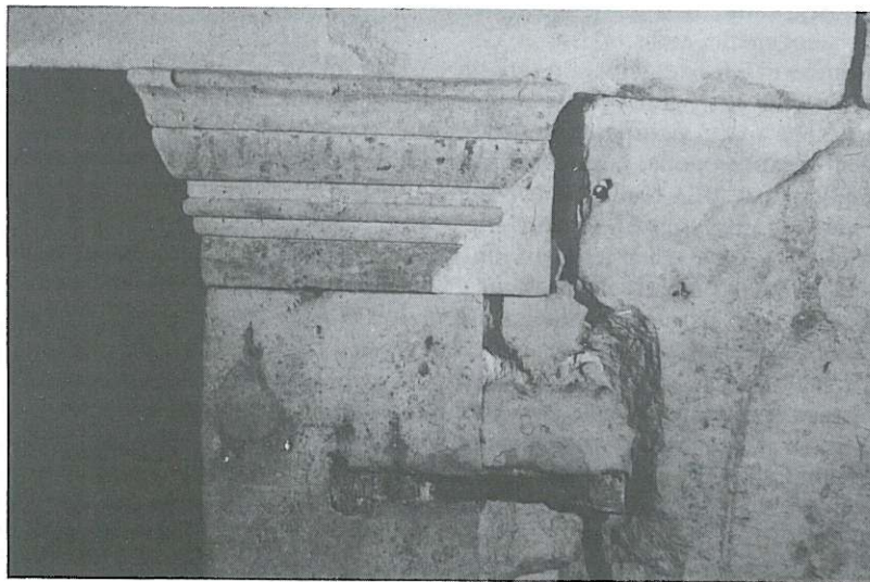
Fig. 8. Eastern pilaster at the entrance of tomb No. 13. The iron brace had been pulled out of place by horizontal strength.
