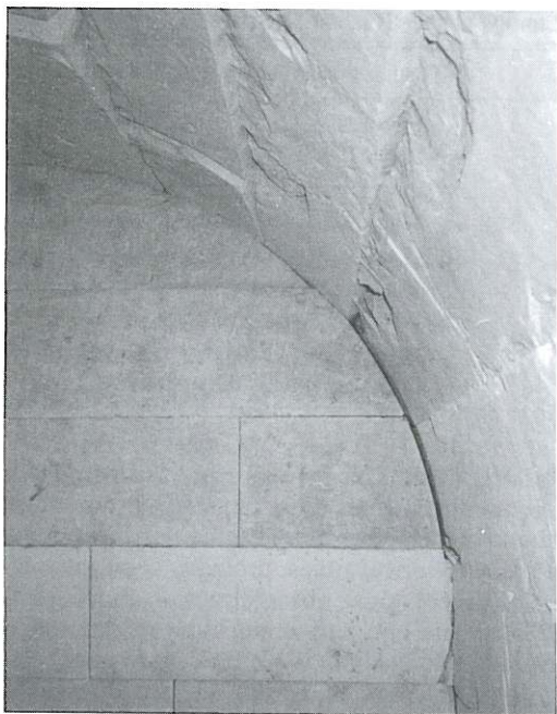
Fig. 7. Flaking of stone blocks as a consequence of the high vertical pressure that they had undergone in tomb No. 13.
