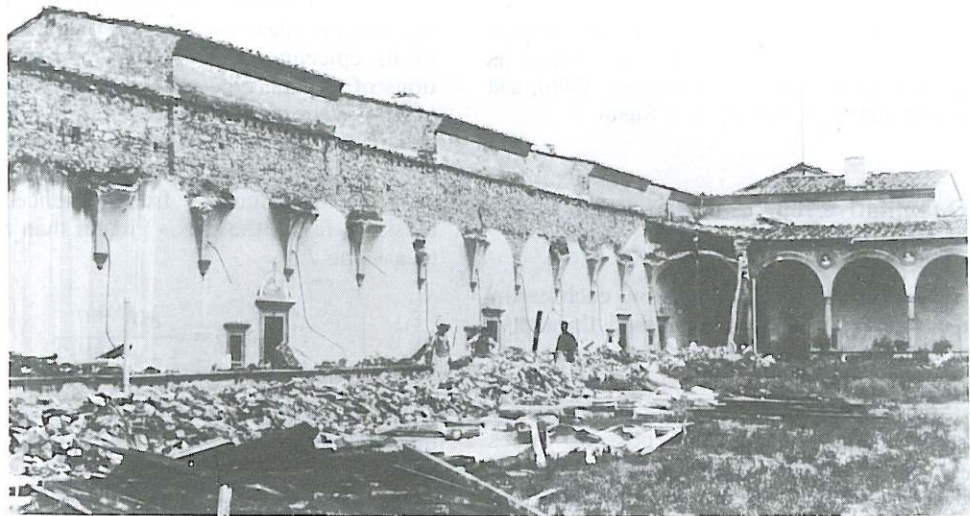
Fig. 9a,b. Effects of the earthquake of 18 May 1895: a) Florence: Spedale degli Innocenti : buttressed front during the restoration works. This building, by Filippo Brunelleschi (1419-26) and completed by Francesco della Luna, is of great importance for the history of architecture in the Renaissance; b) Certosa of Galluzzo: collapse of the north-western end of the great cloister. The building of the 14th century was enlarged during the 16th century. Now it retains a valuable art gallery.
