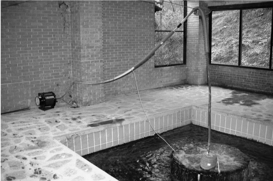
Fig. 4. Station of Tramutola with gas flow meter and the strong gas emission at the thermal-water well.
