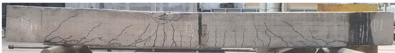
(b) Rupture type of D1: Slip failure at the left end.
