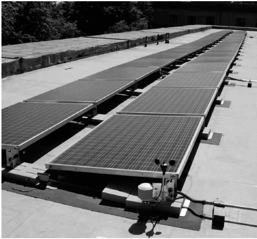
The 12-Kilowatt photovoltaic panels on the roof of the Hayden Library at M.I.T. look impressive but provide less than one percent of the library's daily electrical needs.
