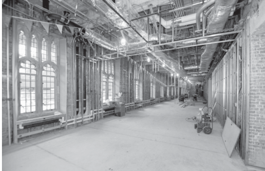
Increasing efficiency by updating building systems was central to LEED certification for the Rubenstein Rare Book and Manuscript Library.
