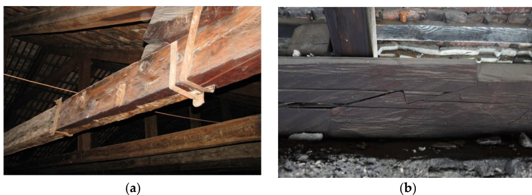
Figure 4. Examples of scarf and splice joining of wooden beams in existing buildings: (a) building in Italy, (b) building in Poland—13th century Czocha Castle in Sucha.
