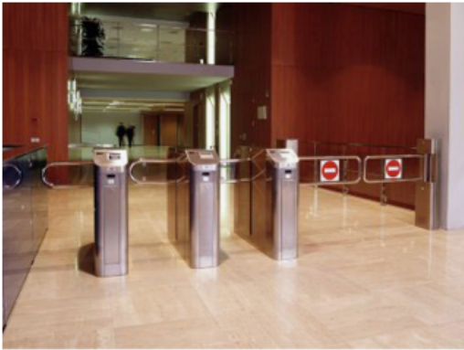
Figure 12: Individual access control.
