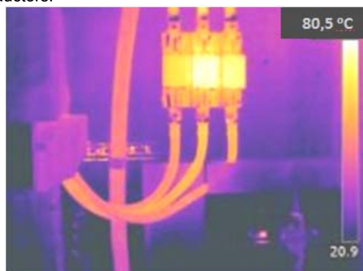
Fig.8 Thermogram high voltage breakers
