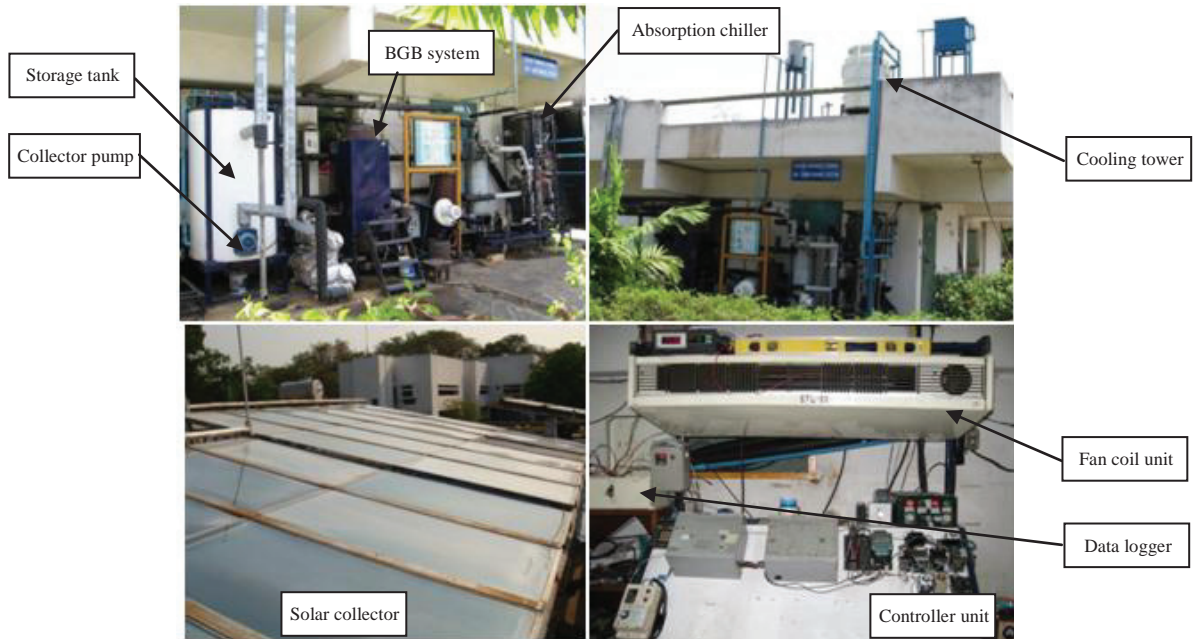
Fig. 2. Fabricated experimental setup of the solar-biomass hybrid absorption cooling system [6]
